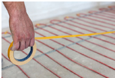
ELECTRIC FLOOR HEATING
