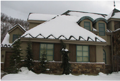
ROOF & GUTTER DEICING
